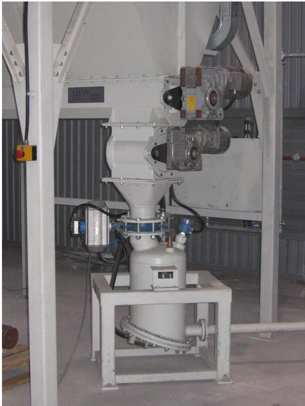
Pneumatic transport dust collector - silo
